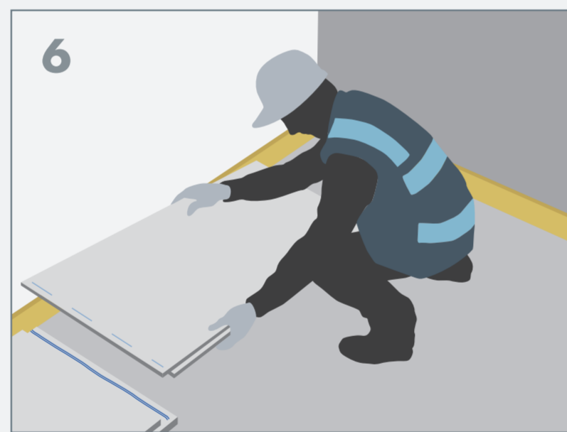
6 Lay the tiered edge of the next board onto the twin bead of adhesive.
