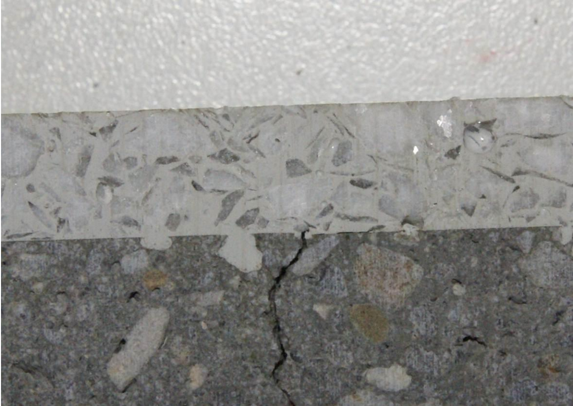
Photo 6, Intact over a 0.5 mm wide crack in the additional test.
