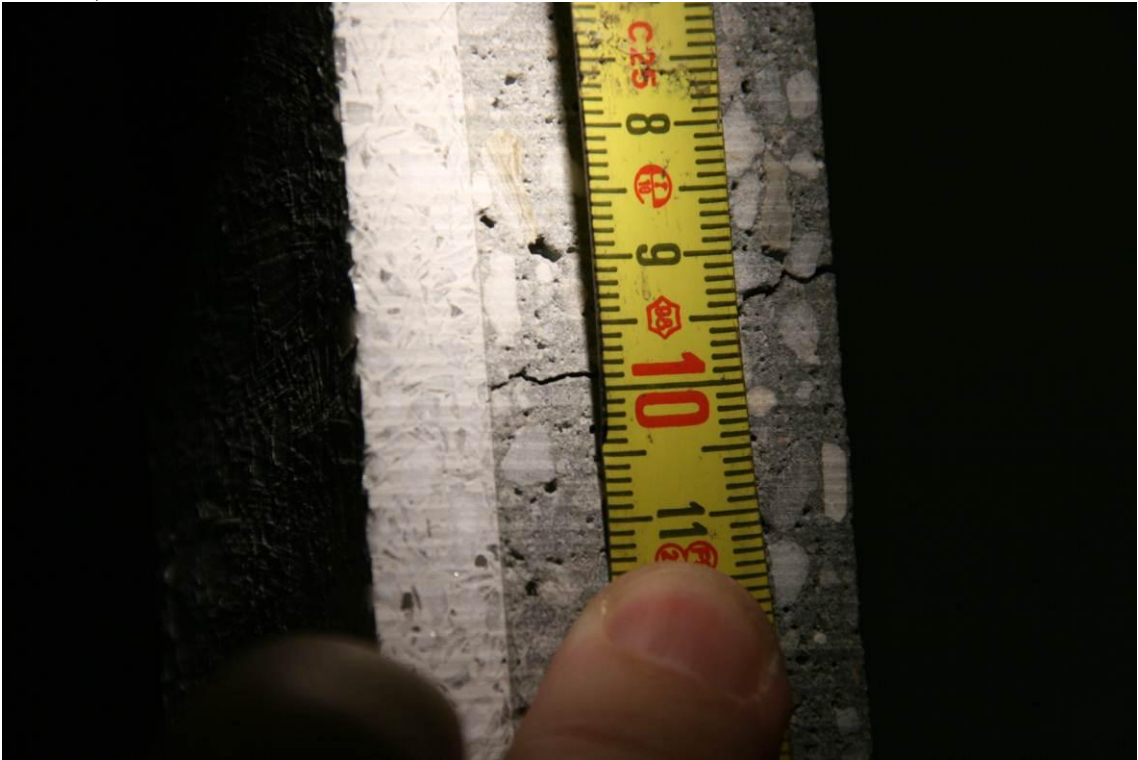
Photo 2, Measuring the width of the crack.
