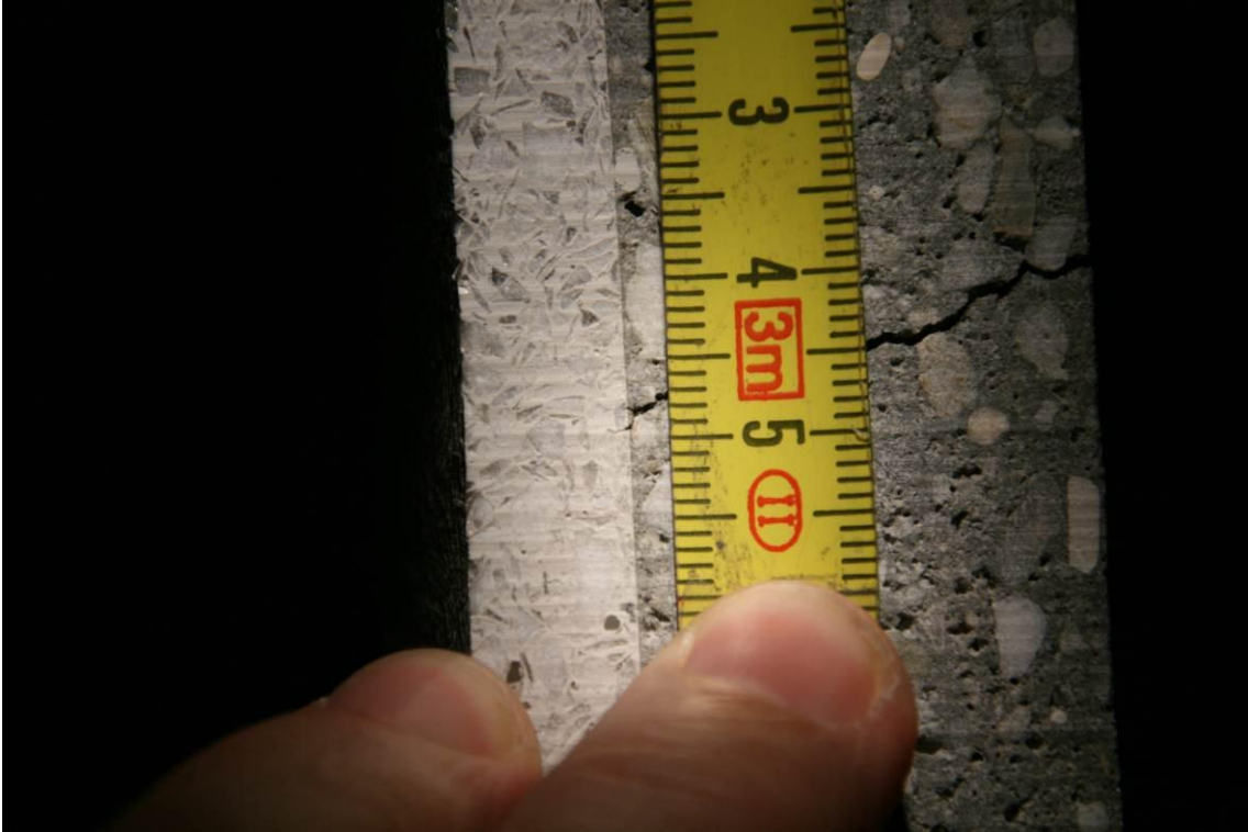
Photo 3, Measuring the width of the crack after extra displacement (approx. 0.4 mm).
